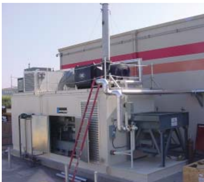
In a beverage manufacturing plant, this critical load support system is designed for combined heat and power (CHP), delivering approximately 70% of the plant's electricity and 30% of its hot water needs.
