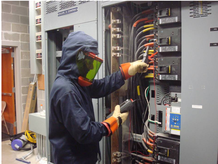
Figure 2: Example of Panel Metering
