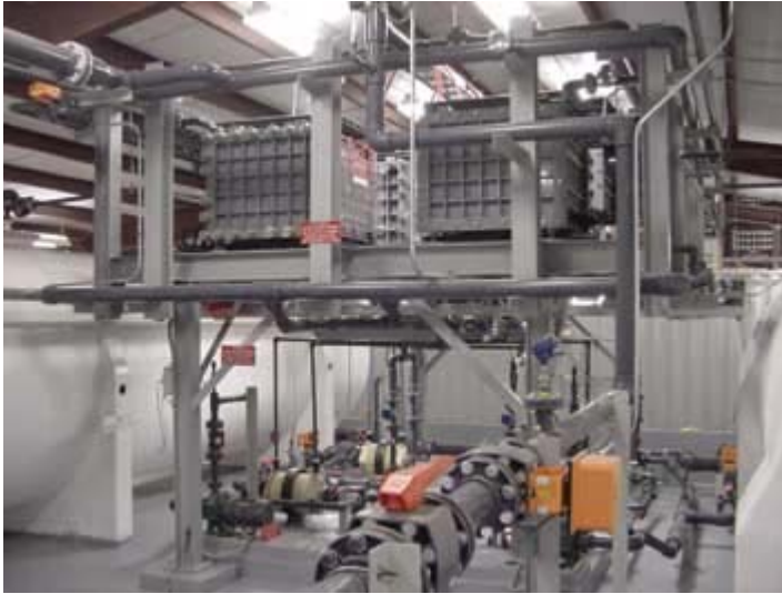
Pipes and pumps carry the vanadium solution to stacks of proton exchange membranes, which transfer electrical charge and create a current.
