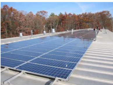
Solar panels funded through Clean Energy Choice low-income matching grant at Western Mass. Food Bank
